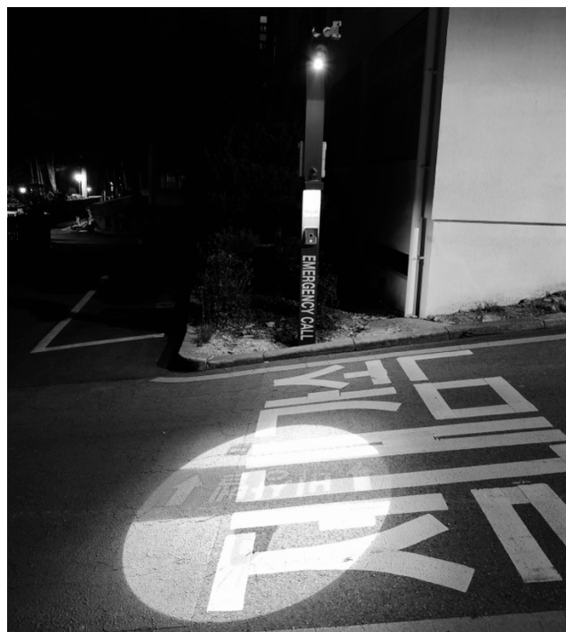
Figure 9. CCTV cameras (top of pole) and emergency button with projection on street to draw attention to the presence of both.
